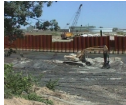
Using sheet steel to help separate and solidify contaminated sediments is a technique used in the Pine River subwatershed.
